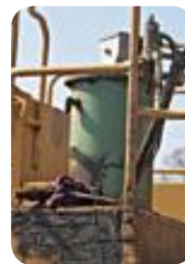
Over-filled reservoir with no overflow prevention system
